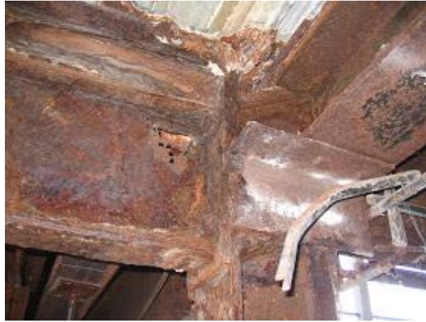
Figure 1.10. A corroded steel beam-to-column connection.
